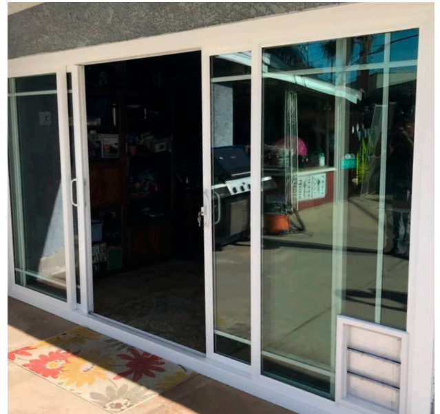
Sliding Patio Doors
